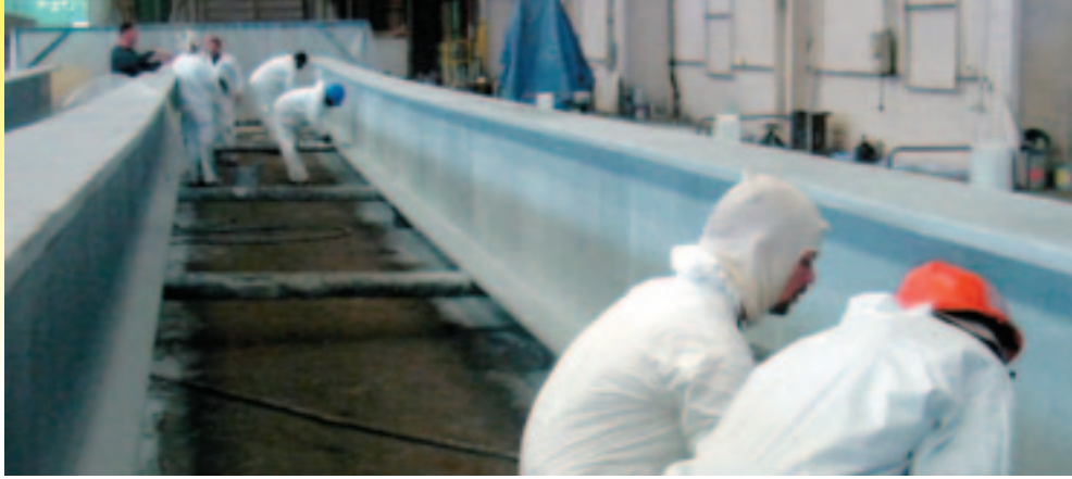
MacKenzie crew members apply Isolatek's Cafco SprayFilm WB 3 intumescent coating on the support beams of a pedestrian walkway in the convention center. The two 480-foot-long, 20-foot-wide skybridges span the exhibit floor and are about 20 feet off the ground.
